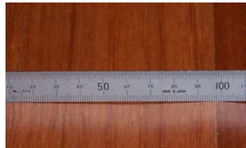
Cupping: board edges higher than the centre of the board
