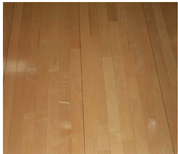
Particularly for wide floors or in moist climates small regular gaps at provide the additional expansion allowance needed. These often close during humid periods.
