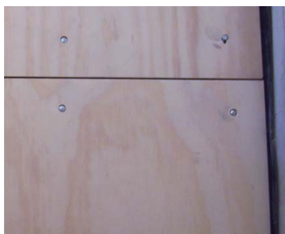
Fixing of the plywood sub-floor through the polyethylene membrane and into the slab
