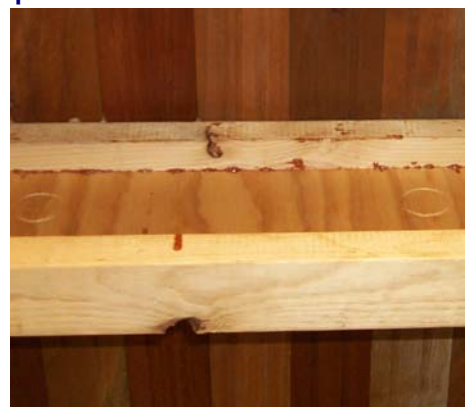
Timber floors are successfully laid over a range of solid timber and engineered joist systems.
