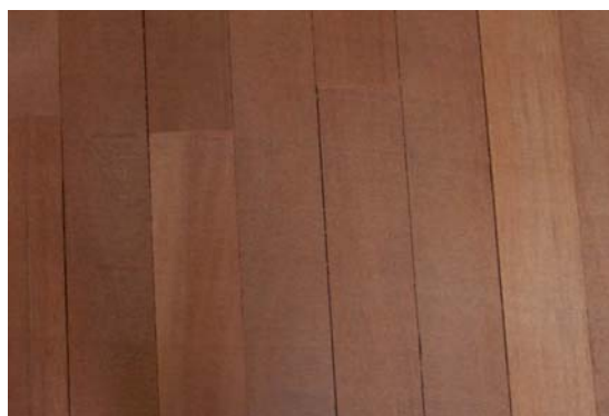
Wide gaps due to high moisture contents at the time of machining.
