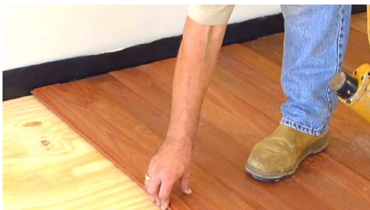
Secret fixing to a plywood sub-floor. A polyethylene moisture barrier has been placed over the slab and both the plywood and flooring are clear of the wall.
