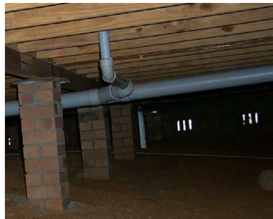
Adequate sub-floor ventilation and a dry sub-floor space are a must for timber floor performance.
