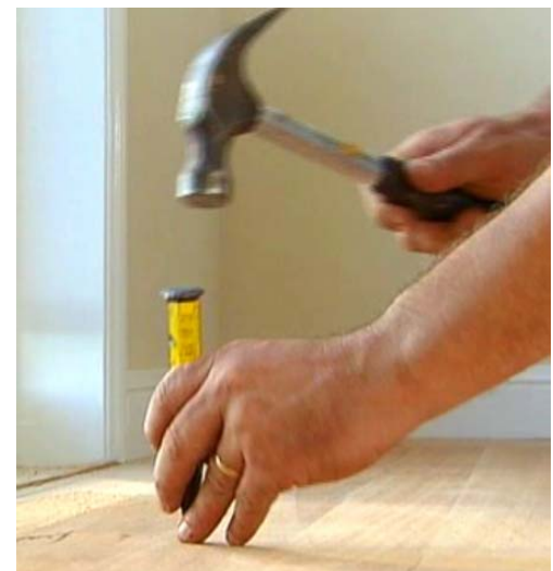
Nails to be punched and holes filled.
